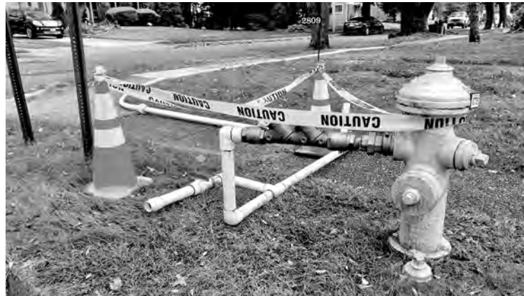
As part of the MPWC's water main relining project, contractors will be placing temporary water lines down the sidewalks, as well as installing temporary service lines to outside hose spigots.
